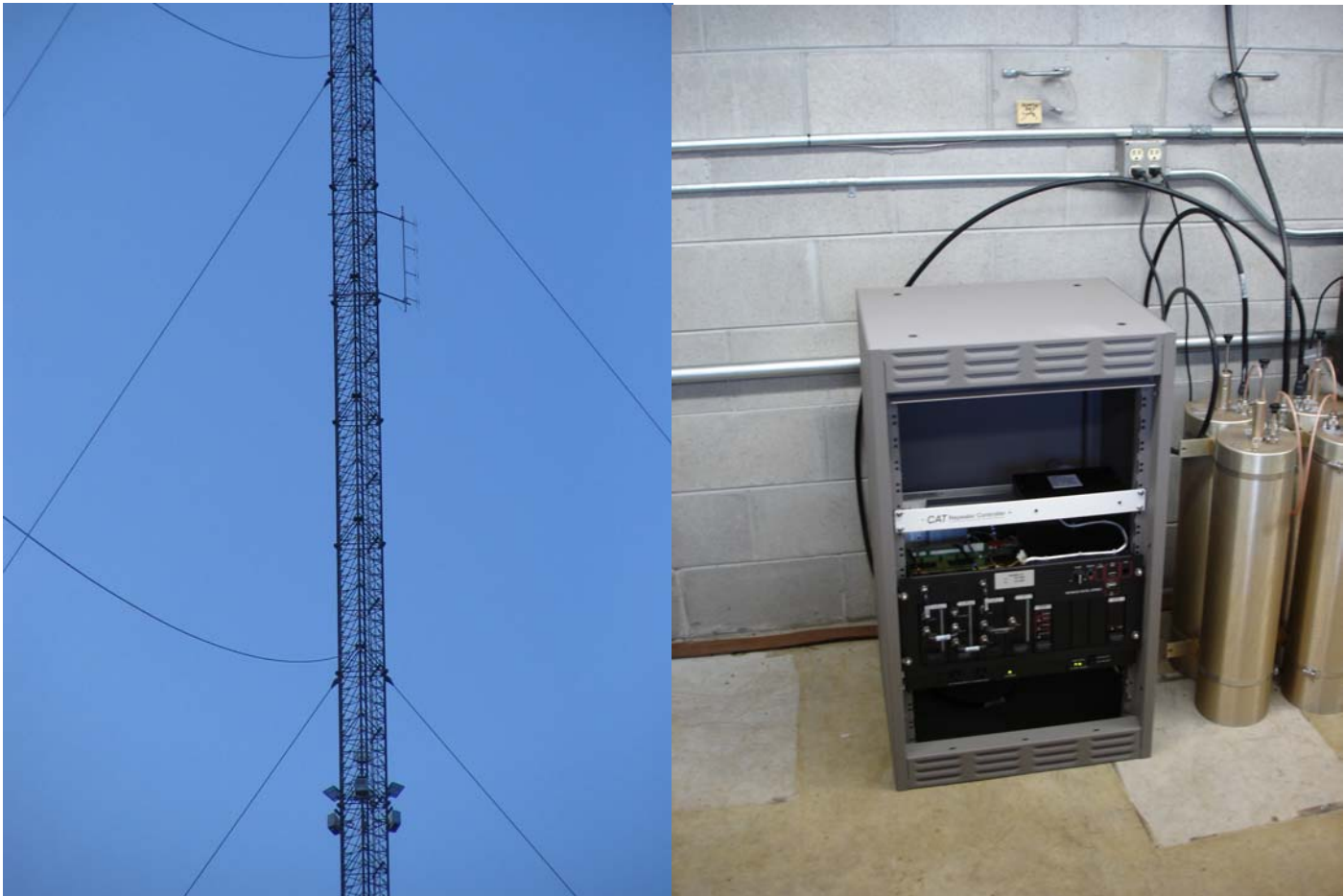
WE9COM Repeater in Suring, WI
