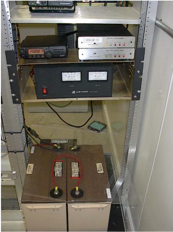
Door County ARES/RACES Packet and APRS Digipeater Emergency Power Configuration
